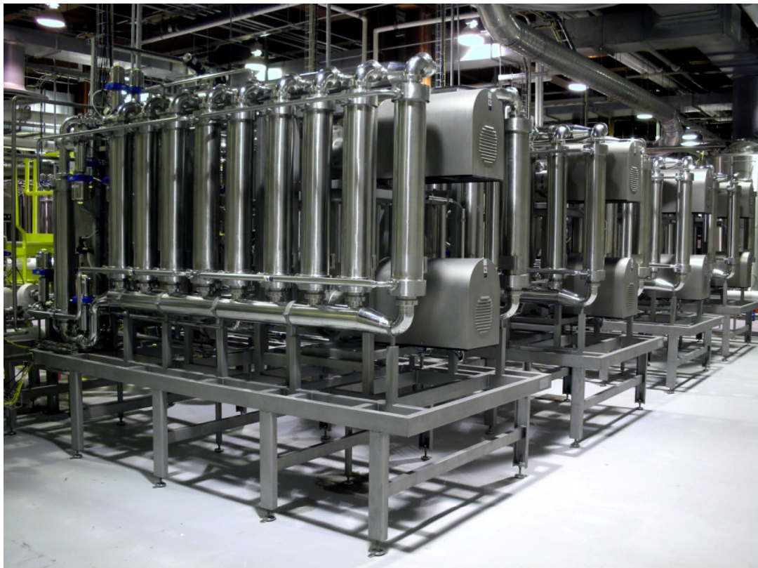
Fig. 1. A recent membrane filter installation (Coors Brewing Company, Shenandoah, Virginia, USA).
